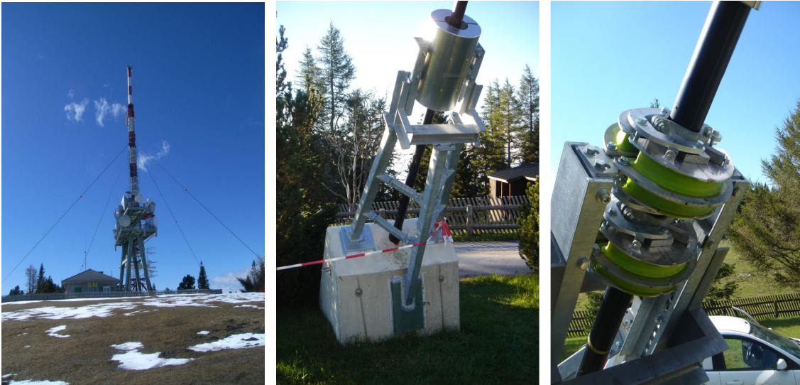
Figure 6: Transmission mast at the Schöckl and stay cable with installed damper
